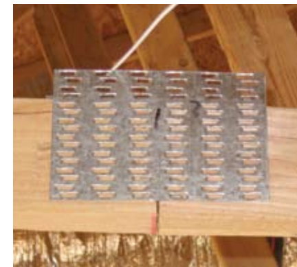
Figure 1. Plate misplacement. Engineering specified bottom edge of plate at the bottom edge of the chord.
