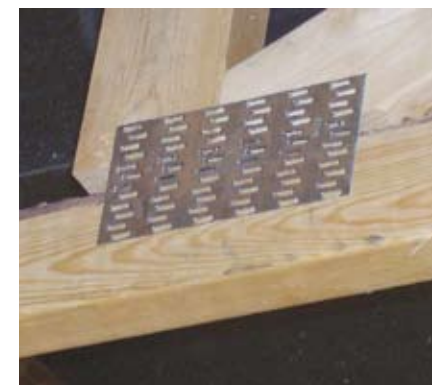
Figure 3. Wane under plate contact area of bottom chord.
