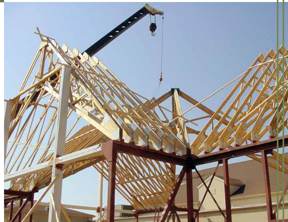
Photo 1. After the steep half scissors trusses were assembled on the jobsite, the trusses for each of the four legs of the addition were set by crane. Steel beams along the top of the walls of each leg and glulam beams in each of the four gables resist horizontal and vertical forces.
