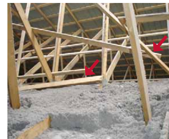
Photo 1. Example of broken compression webs in which the CLR was attached but had no diagonal bracing. The red arrows point to the broken webs in two adjacent trusses. Note that the CLR is still attached to one of the webs.
