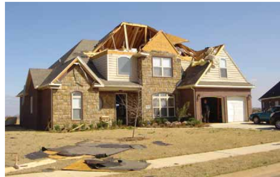
Tornado damage exposed framing issues that revealed structural defects in this home.
