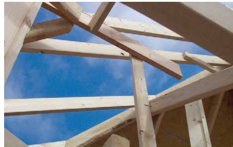
The end of a ridge beam for a dormer is bearing on a 2x4.
