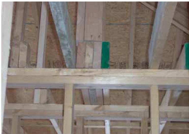
Spradlin says examples of poor framing practices can be found in his market. For example, in this photo, a 4-ply beam bearing on a wall has no studs under it to transfer the load to the floor below.
