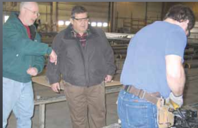
Ray Jr. demonstrates how screws are fastened into the heel of a steel truss.
