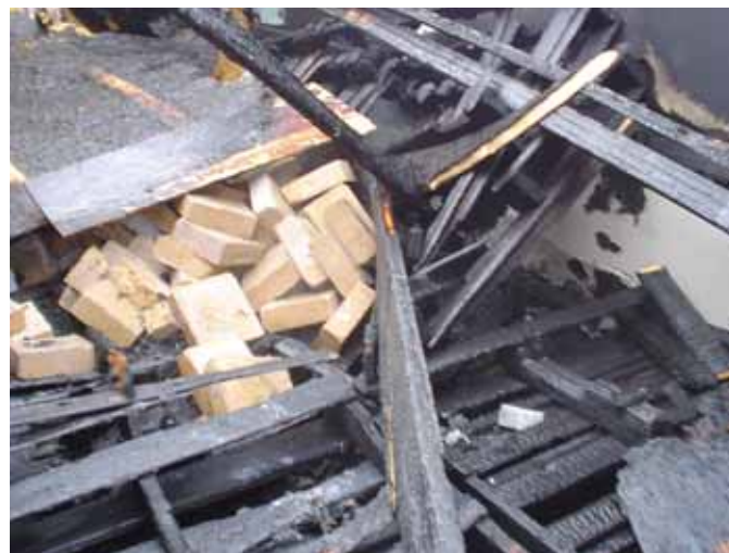
After the fire, severe charring was seen on all structural members. Even on the outside truss, charring reduced the size of the chords significantly. Without trying to make this point, the demonstration also showed the effectiveness of gypsum protection on the walls.
