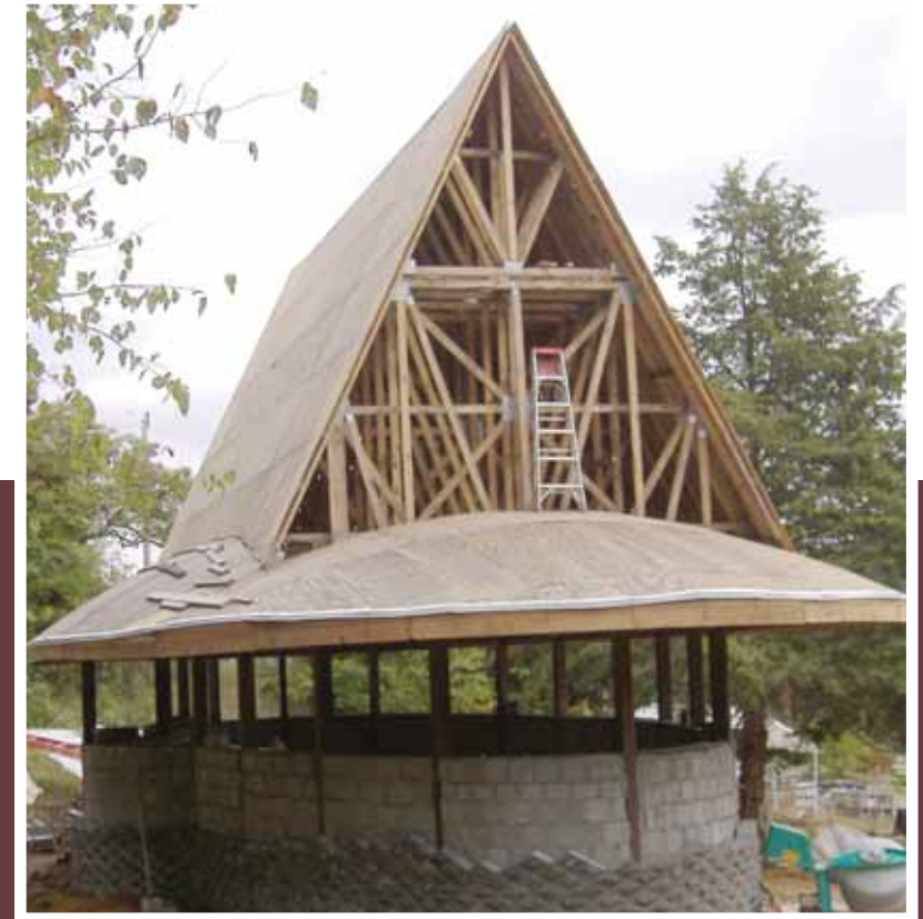
The roof's curved shape made designing the trusses using conventional design software extremely difficult.
