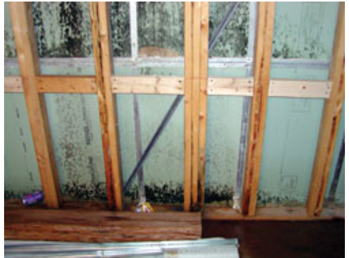
Figure 2. Extensive mold growth on paper facing of gypsum board in fire wall between adjoining town homes. Minimal mold growth is present on the wood framing. Roofs between these two units had not been sealed allowing rain to penetrate the enclosure and wet this wall. (Photography by Nathan Yost, Building Science Corp.)
