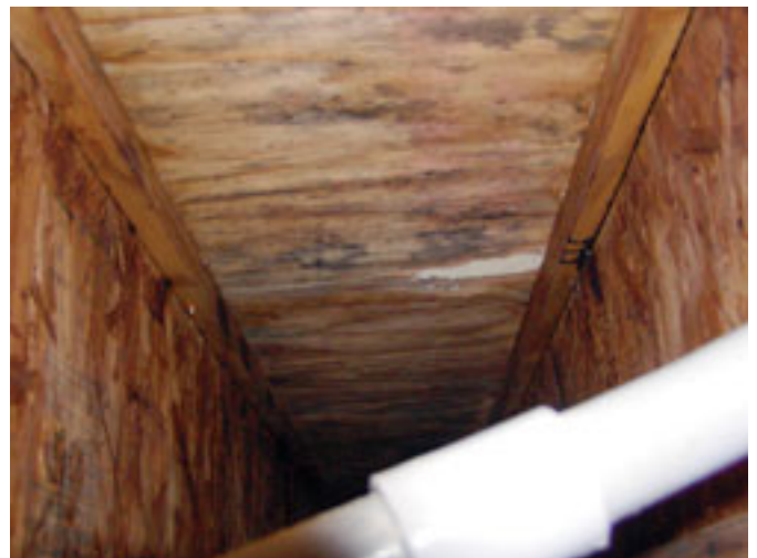
Figure 1. Mold in crawl space during construction. The underside of the floor sheathing and the I-joists have elevated moisture contents (25-30 percent by weight) as well as mold growth. Rain collected on the crawl space floor providing a
