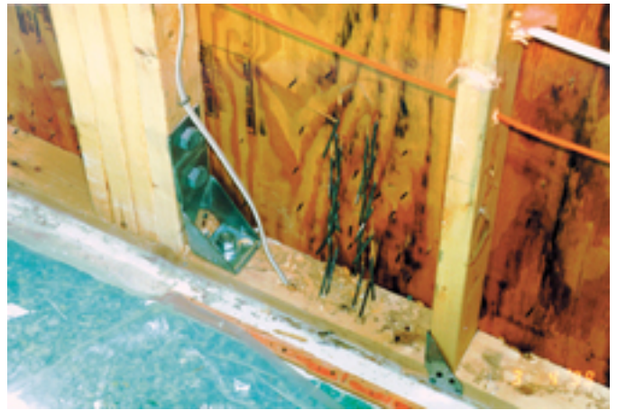
Figure 2. This connection has several problems. The four studs were not nailed together to act as a unit, and the horizontal bolts were loose due to oversized holes.
