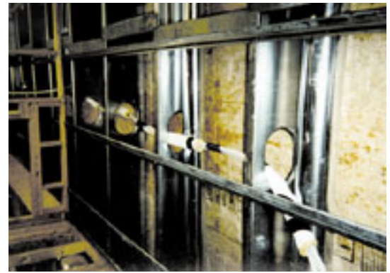
SINCE THESE JOISTS WERE SPACED 32" APART, IT WAS NECESSARY TO ADD HAT CHANNEL FOR HANGING DRYWALL
