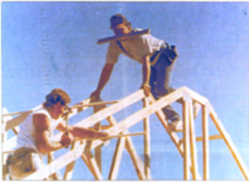
Easy does it While framing, there's a danger of overloading the trusses with a heavy, solid board. Instead, all the trusses being connected to a truss at their top should be braced with a spacer. This is the best way to do it.
